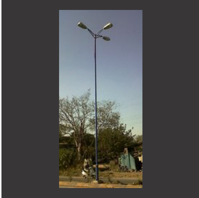
Street Light Poles
