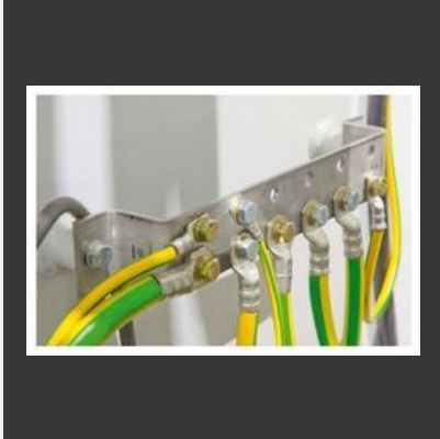
Earthing and Lightning Protection
